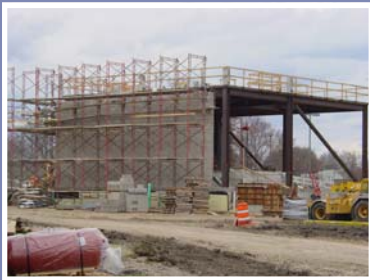
ISJ/Mayo Health Systems Power Plant, Mankato, MN
